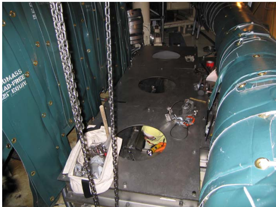
Ecomass Blankets in use at Sequoyah Nuclear Plant
